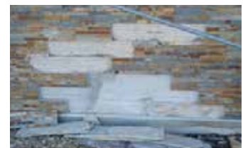
Delamination of Stone
